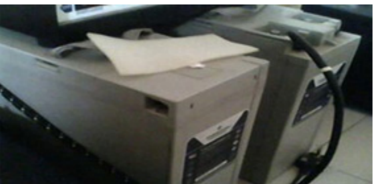
APPENDIX 4 - Two Emerson® 50 Ampere Deep-Cycle Batteries
